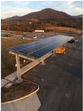
New Solar Canopy
