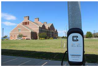
Electric Car Charging Station
